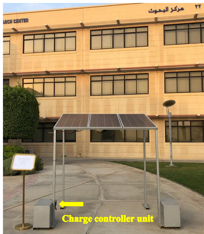
Figure 4.2: Implemented solar carport.
