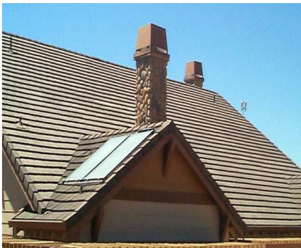
Figure 3.2 - solar panel installed on rooftops
