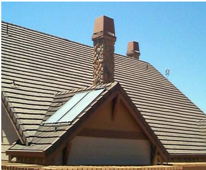
Figure 3.2 - solar panel installed on the roof of a house
