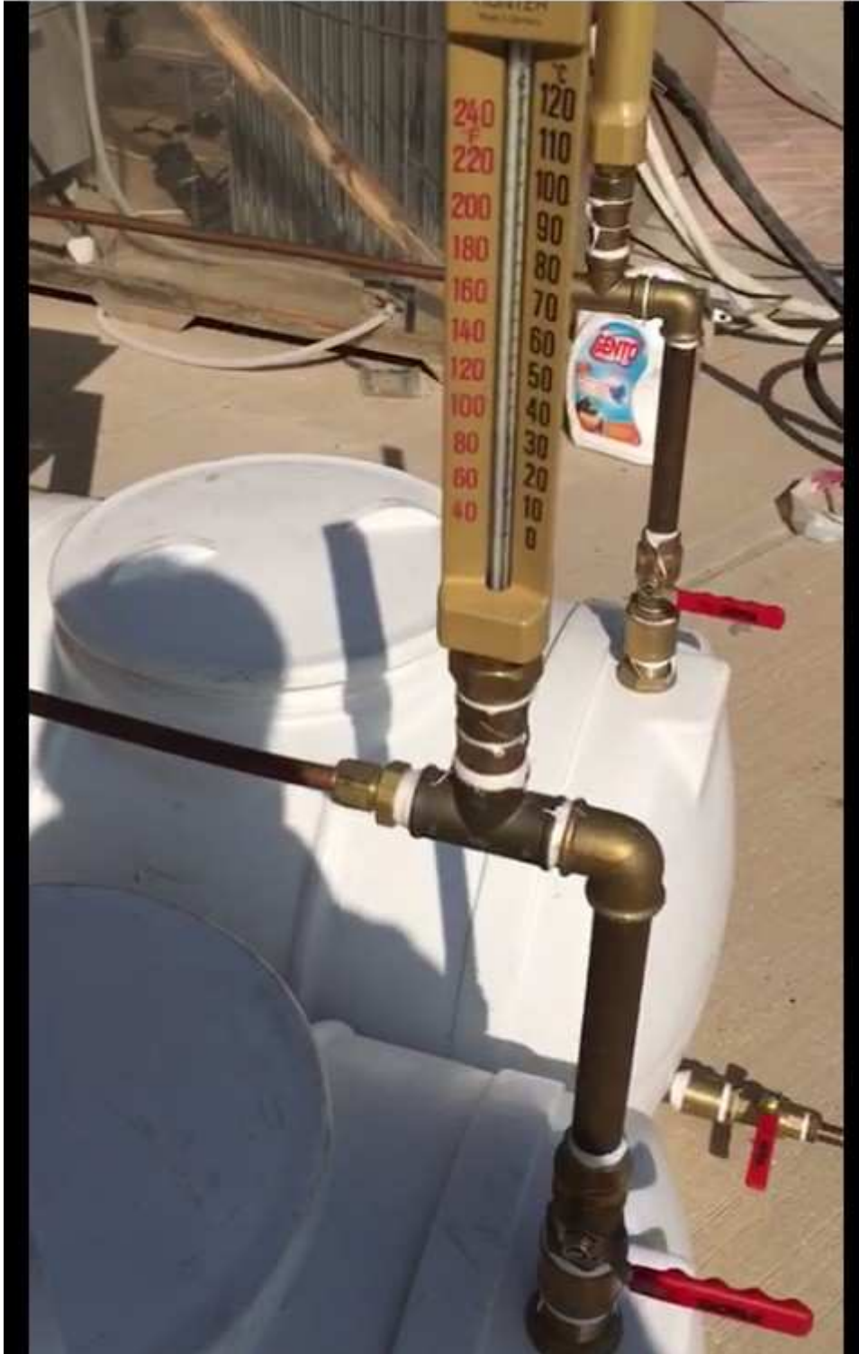
B.5 the outlet tanks and the outlet thermocouples
