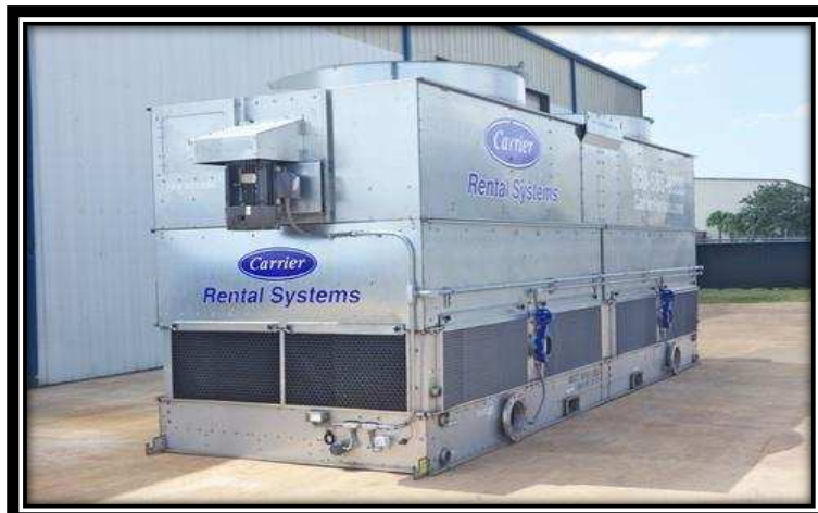
Figure 1.2 A/C cooling tower
