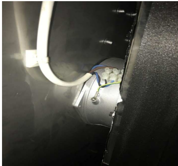
Figure (3.6): The exhaust fan.
