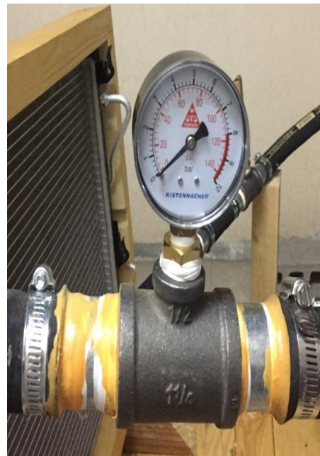
Figure (3.15): Pressure gauges
