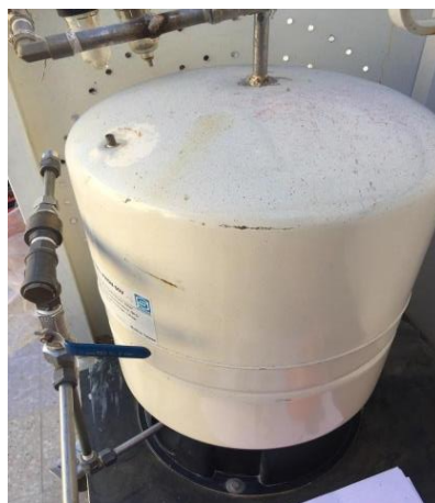
Figure 3.10 (The Pressurized Tank We Used)
