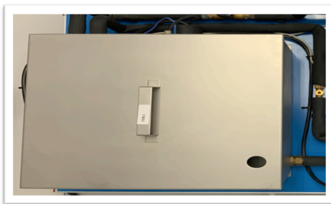
Figure 3.2.3.1a: Hot water tank
