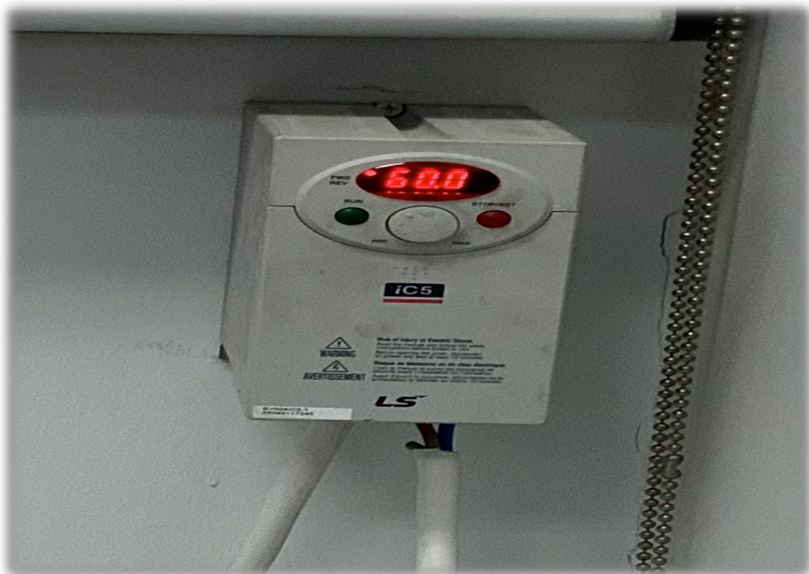
Figure 3.7.3: Variable frequency drive (VFD).
