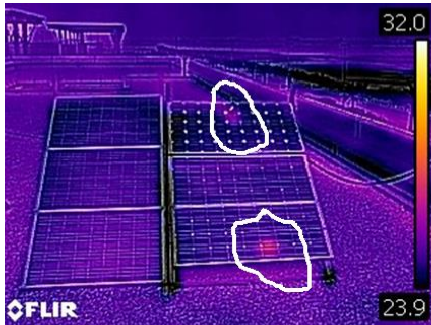
Figure 13a General Failure PV Panel
