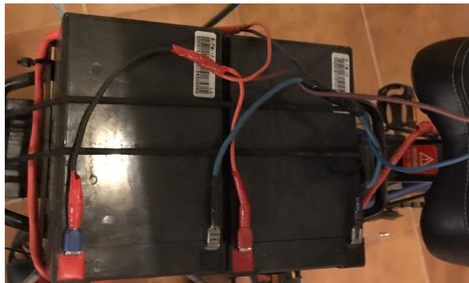
Figure 4.16: Batteries connected in parallel
