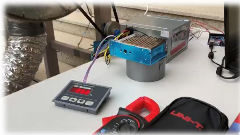
Figure 24 - Speed Controller & Amp Meter
